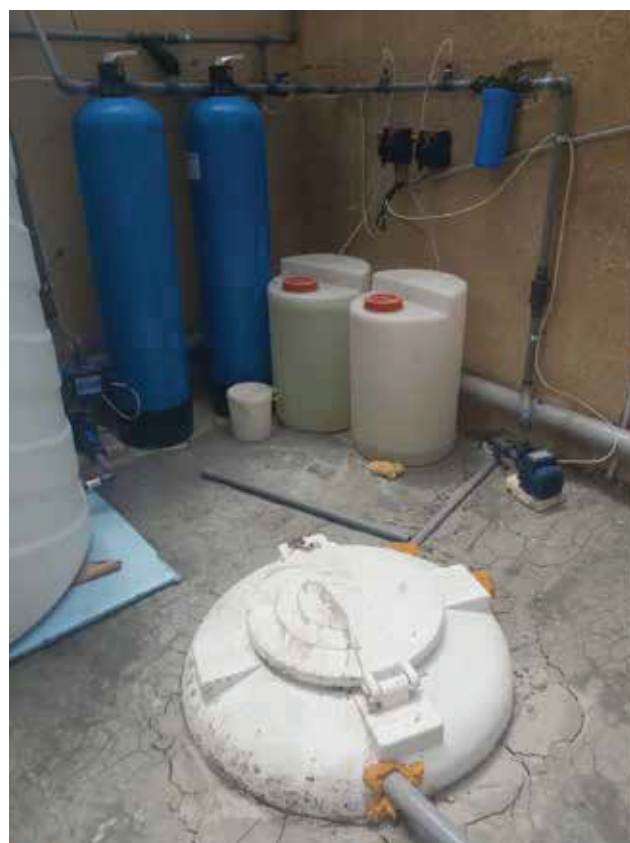
The greywater treatment system installed on site, which consists of physical and chemical treatment stages.
